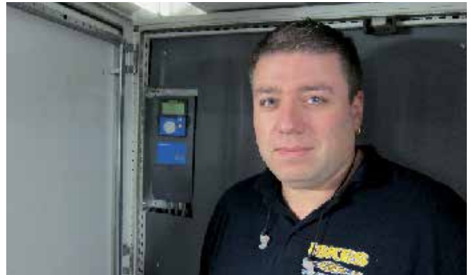
Chief engineer, Guy Knorr, in front of the VACON® NXP Liquid Cooled Drives
